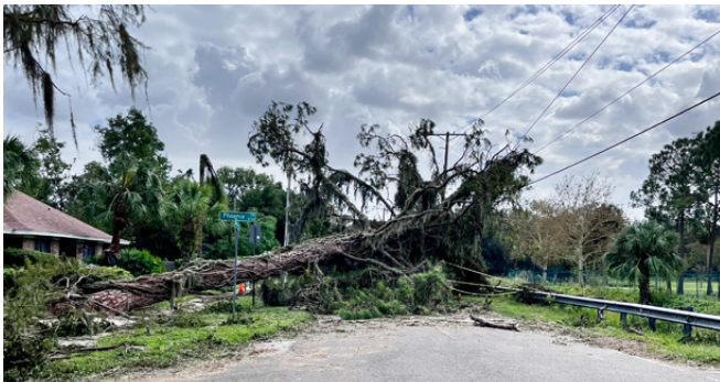
Tree and utility line damage from Hurricane Milton at Phoenix Circle and Orange Grove. October 10, 2024. Photo by Daniel Francis
